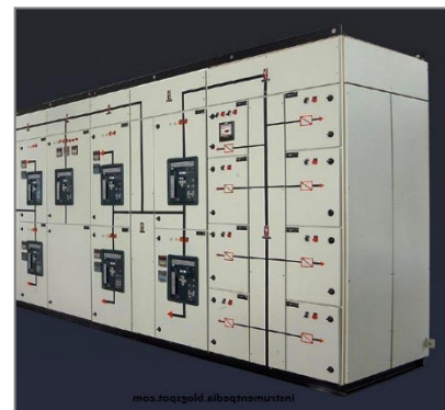
Figure 10: Motor Control Centre
