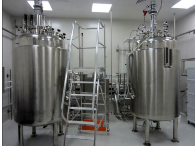
Figure 4: Stainless Steel Tanks
