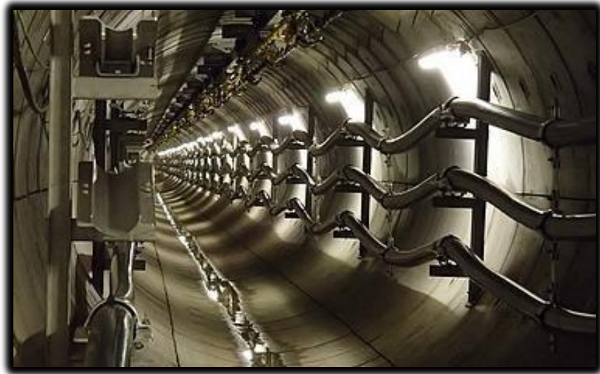
Figure 16: HV Underground Cables
