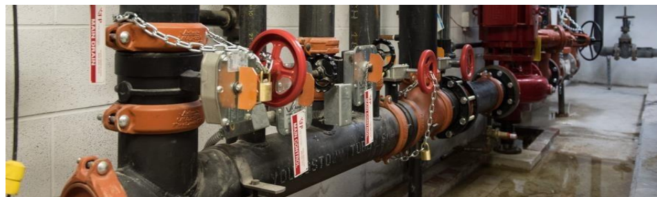
Figure 42: Quell Fire Sprinkler System
