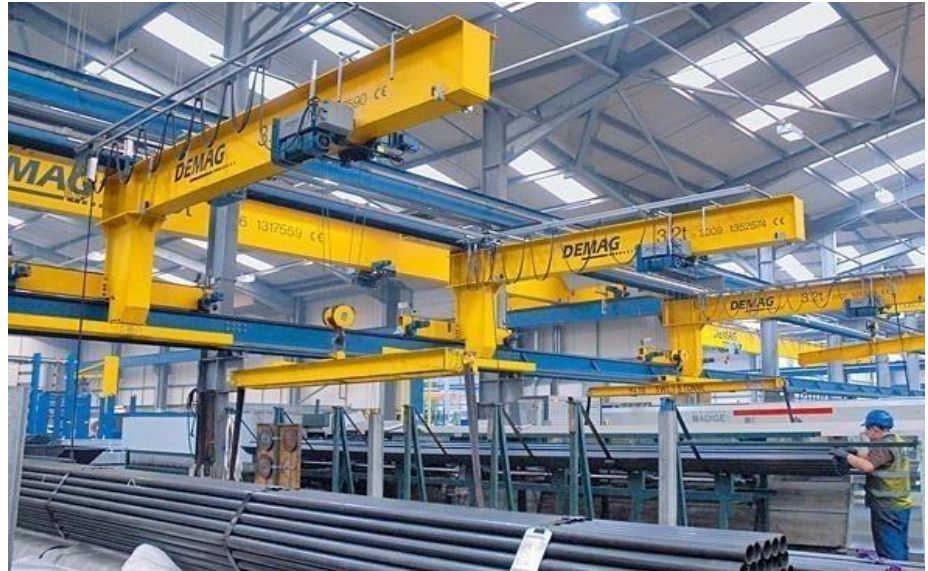
Figure 61: Wall Travelling Cranes
