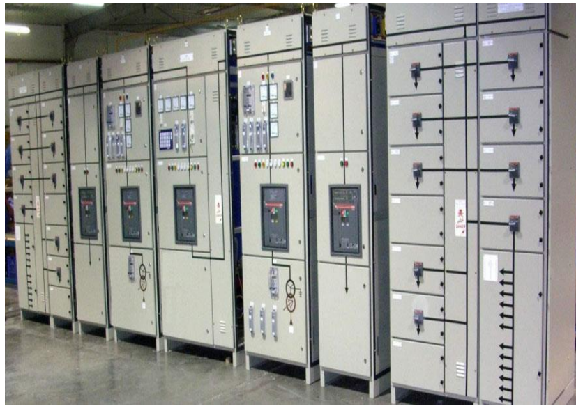
Figure 4: Main Distribution Board (MDB)
