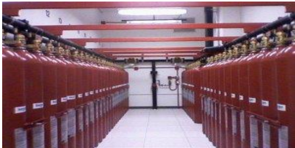
Figure 46: CO2 fire suppression systems
