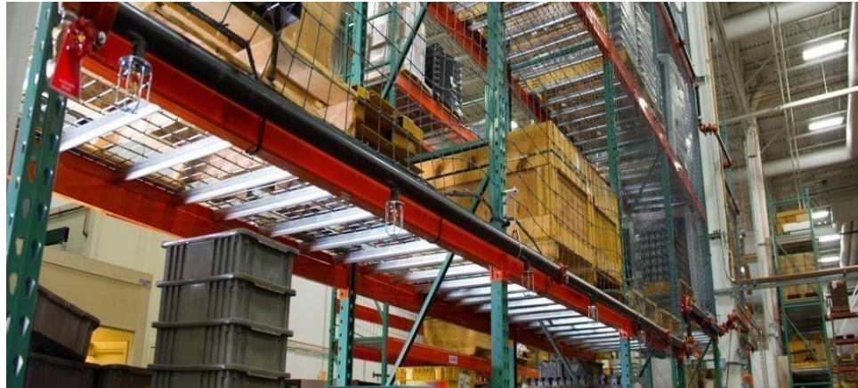
Figure 41: In-Rack Sprinkler System
