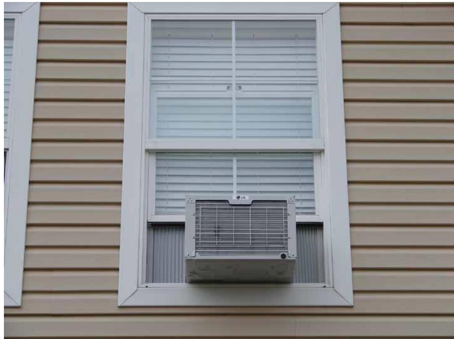
Figure 25: Window Air Conditioning Unit
