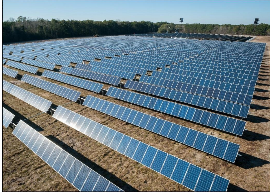
Figure 7: Solar PV Plant
