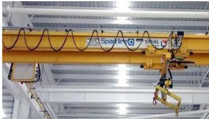
Figure 58: Double Girder Under-Slung Crane
