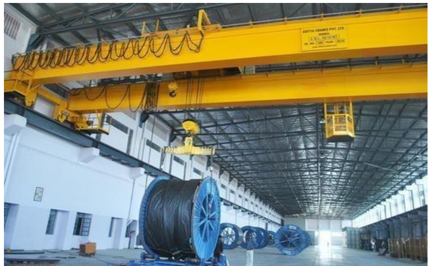
Figure 56: Double Girder EOT Crane
