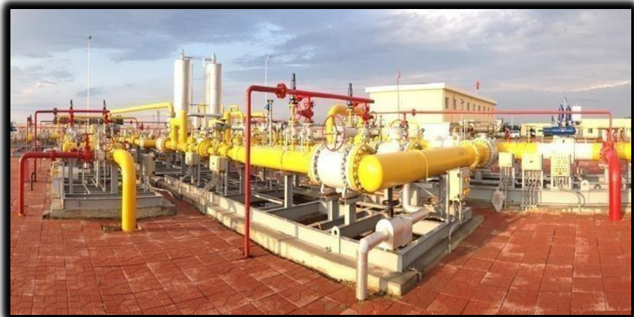
Figure 31: Gas Pipeline, Metering and Regulating Stations
