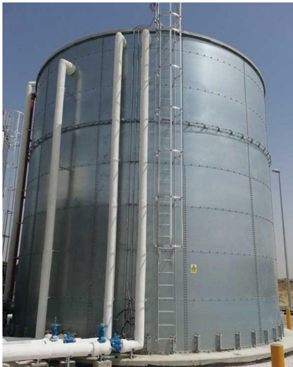
Figure 12: Carbon Steel Water Tank
