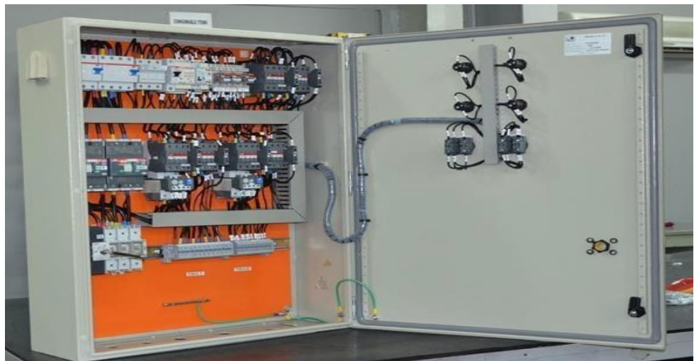
Figure 5: Sub-Main Distribution Board (SMDB)
