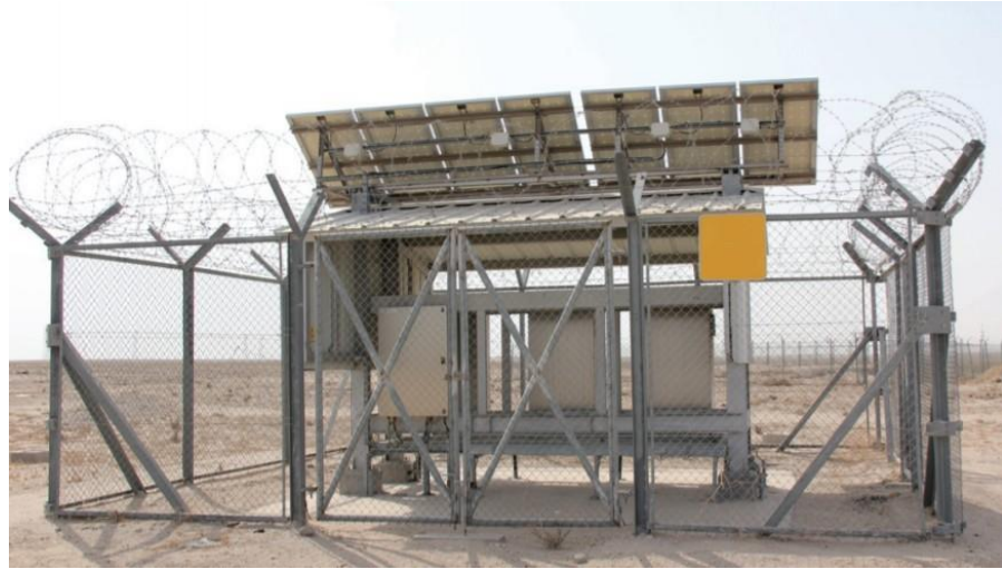
Figure 85: Remote Terminal Unit (RTU) Cabinet for block valve station in the desert
