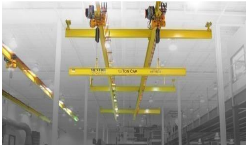
Figure 52: Straight Monorail Cranes
