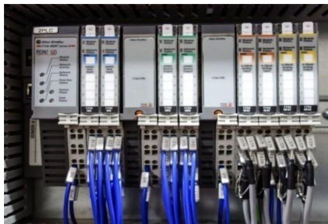
Figure 86: Programmable Logic Controllers (PLCs)
