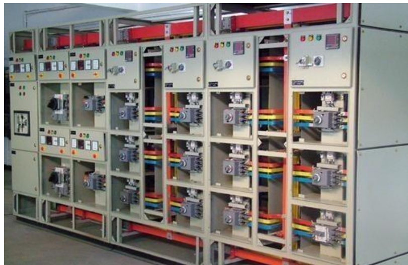
Figure 3: Motor Control Center (MCC)
