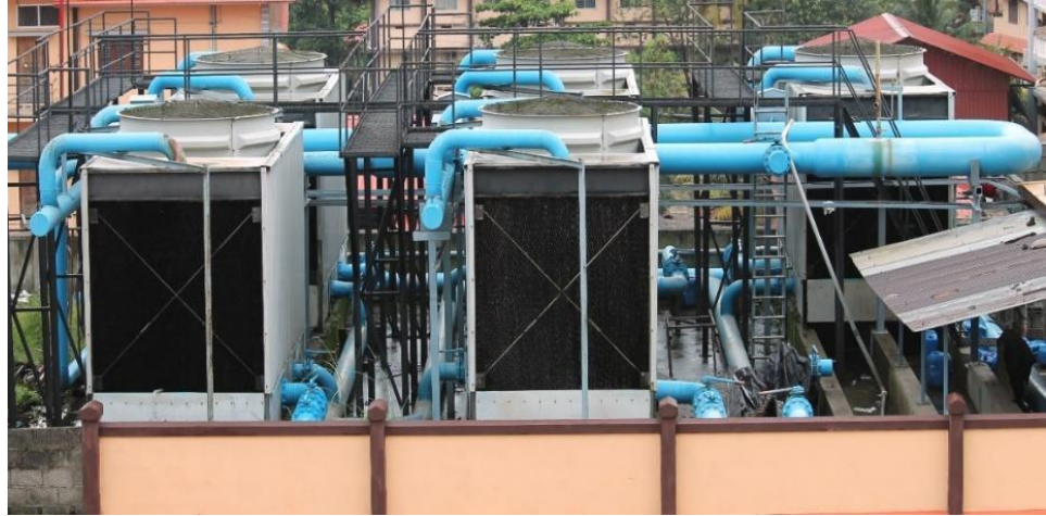
Figure 30: Centralized Air Conditioning Equipment
